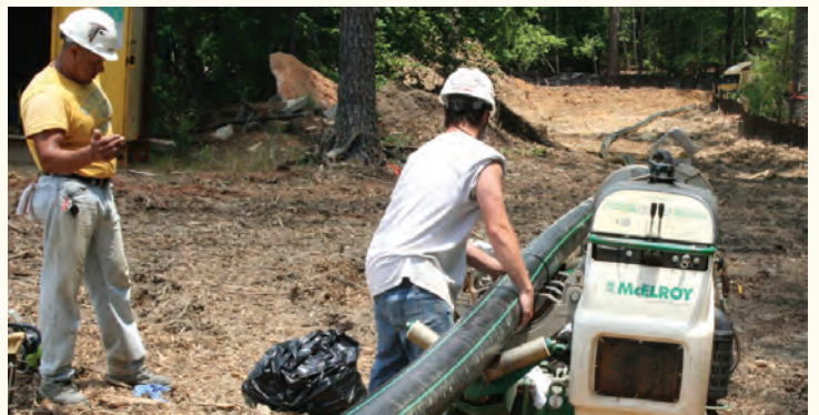
PCWASA contractors from Willow Construction work toward the recent completion of the Meade Field Pump Station project, which included installation of 2,400 linear feet of 8-inch PVC gravity sewer line and more than 4,500 linear feet of 6-inch HDPE force main.
