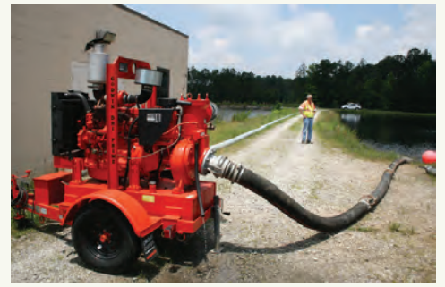
PCWASA Construction Manager Nathan Brooks (background) oversees the removal of water from the Crosstown Water Plant lagoons for wastewater treatment.
