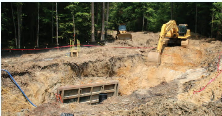
Thanks to the Series 2013 bond issue, which freed up approximately $1.15 million in reserve, PCWASA has additional capital for system upgrades such as the Meade Field Pump Station (above).
