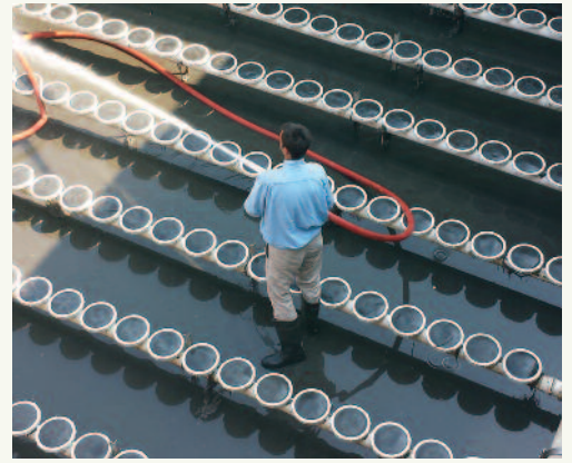
The net cash provided by operating activities, which was a little more than $4.6 million this past fiscal year, provides dollars for PCWASA to reinvest in its sewer system. Resulting system improvements have included rehab to the Rockaway Plant (above), where basins were cleaned to prepare for the installation of new diffusers.
