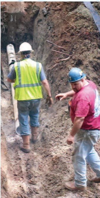
An example of urgent repairs for the PCWASA system made easier because of the Authority’s Annual Services and Emergency Services Contracts is the rehab work on an 8-inch sewer line at Commerce Drive (above).
