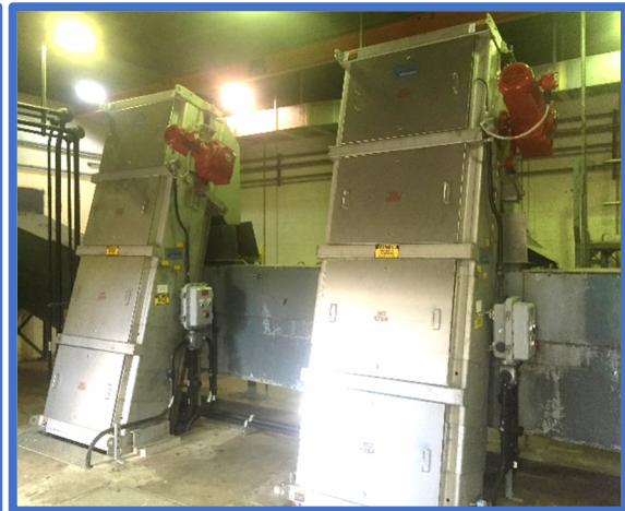
Flagstaff, AZ – Wildcat Hills WWTP – VMR-40
