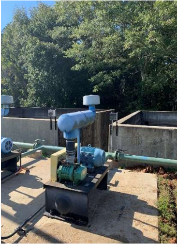
Digester at LC
