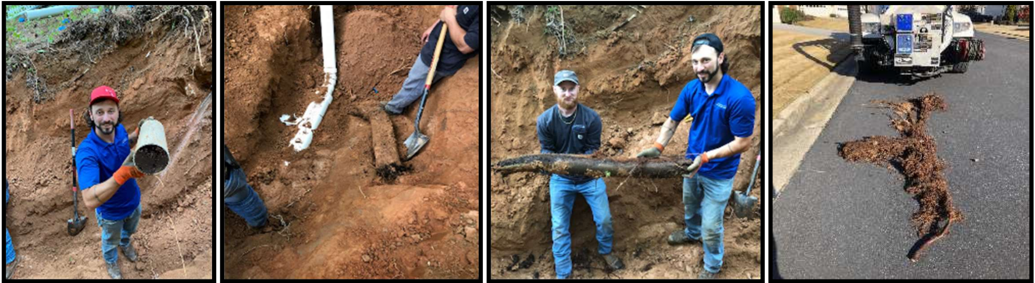
Customer lateral block and line blockage.
