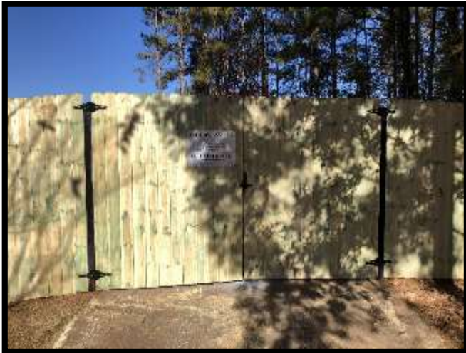
Lift Station 27 Fence
